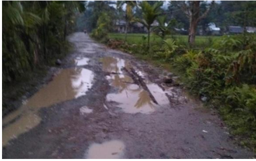
Figure 1. Severely Damaged Road Conditions
